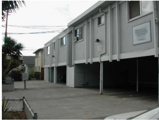
Figure 2. Photo of a typical soft-story multifamily dwelling (MFD) showing the open parking level and upper levels that are more rigid due to the partition walls in the living units. (Photo by I. Syed)
