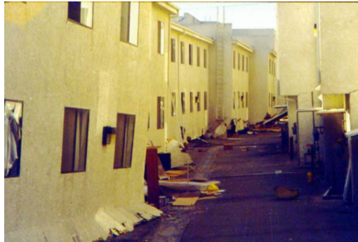
Figure 3. Damage to two tuck-under parking buildings in the 1994 Northridge earthquake. (Photo by G. S. Selvaduray)
