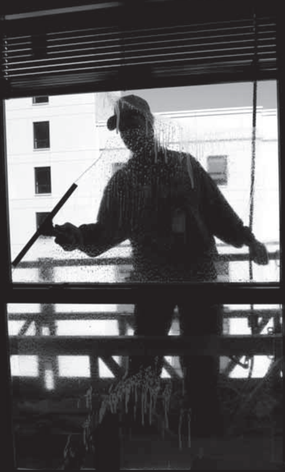
Jose Madris, a JT Window Works employee, washes an exterior, eighth floor window at Campus Village Building B while on a suspended scaffold Tuesday. MIKE ANDERSON / Spartan Daily
