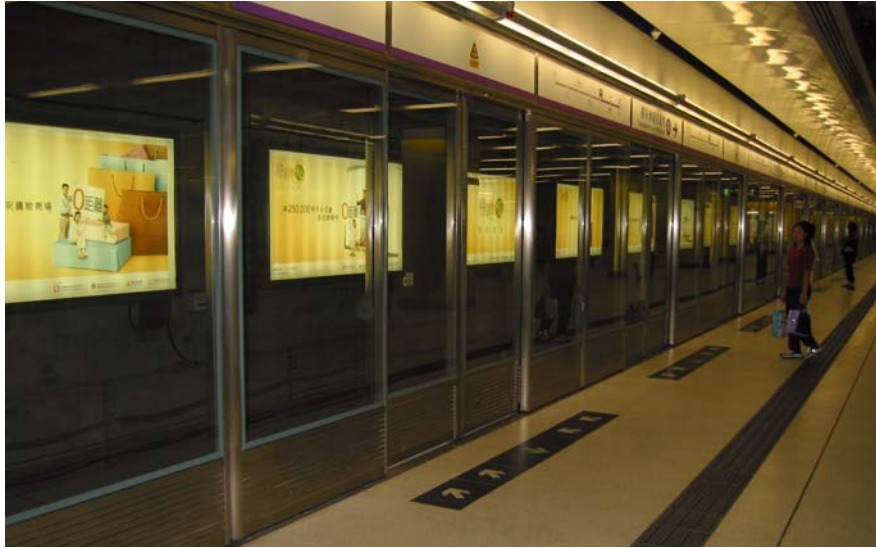
Figure 15 Platform Edge Doors, Hong Kong
