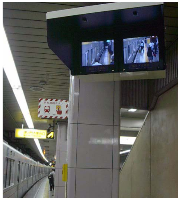
Figure 21 CCTV Monitor, Kasumigaseki Station, Downtown Tokyo
