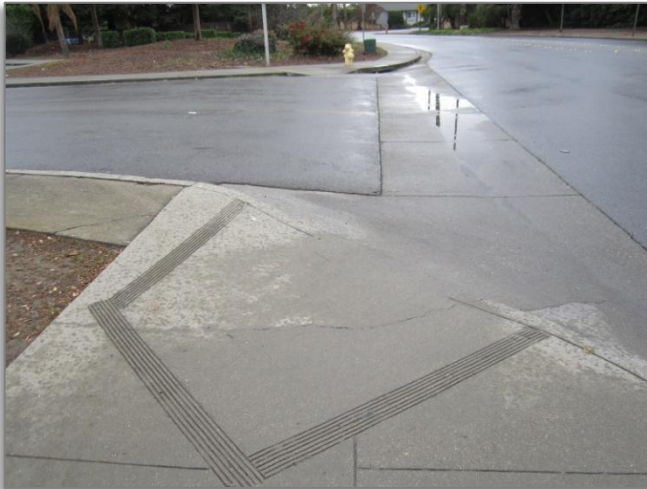
Figure 12. Break in sidewalk due to commercial driveway.
