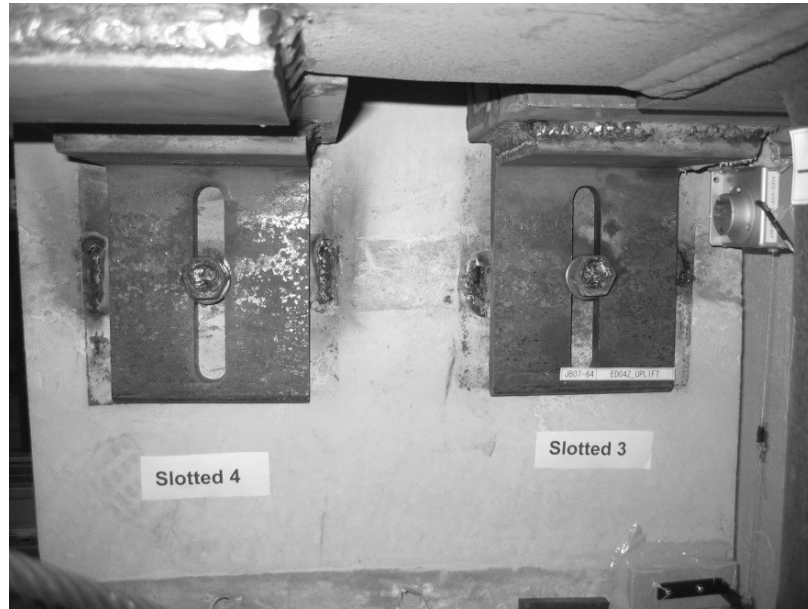
Figure 4.3. Slotted Connections at Top of Panels at 5th Floor (Photo credit: Maggie Ortiz, 2011)
